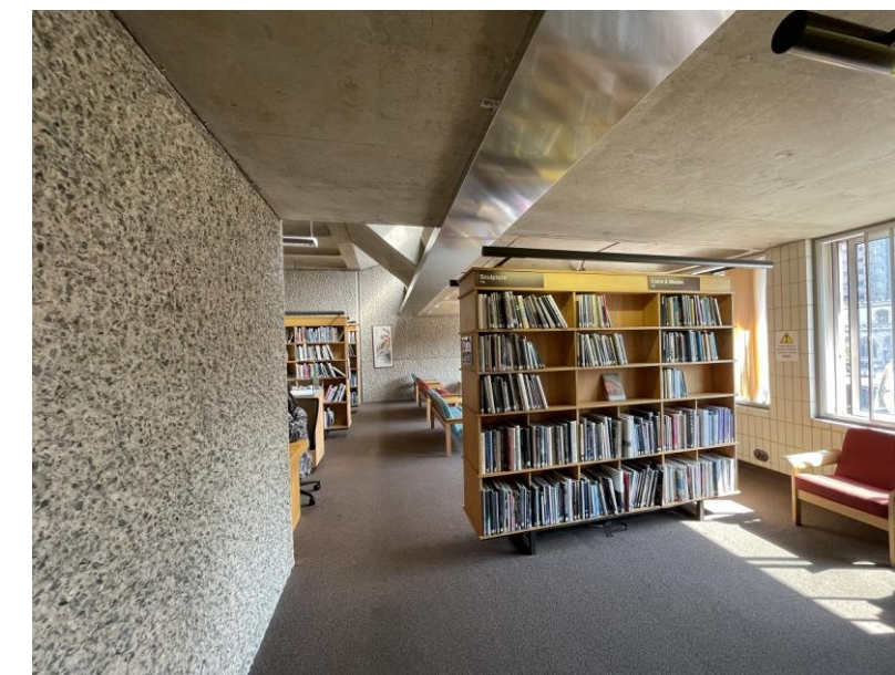
The existing area of soft seating and the proposed location of screen and door D05. The stainless steel tray is an ad-hoc internal rainwater gutter until the external waterproofing of the building is resolved.
