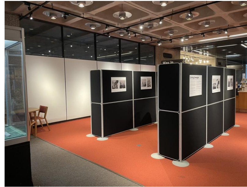
Existing Library exhibition space/foyer displaying 'Living Lineages' photography exhibition and solid, white display panels to metal screen behind. Door D02 to be formed in left hand panel.
