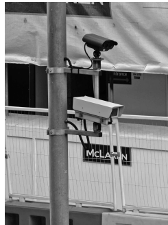
A CCTV camera on Aldersgate, part of the “ring of steel” around the City
